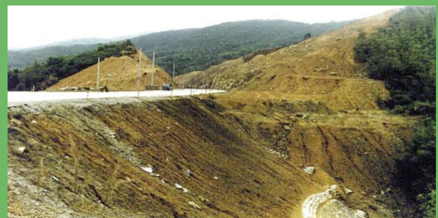
China - unstable highway fill prior to VS treatment. Road stability was so bad in untreated state that major lateral cracks in the pavement occurred
