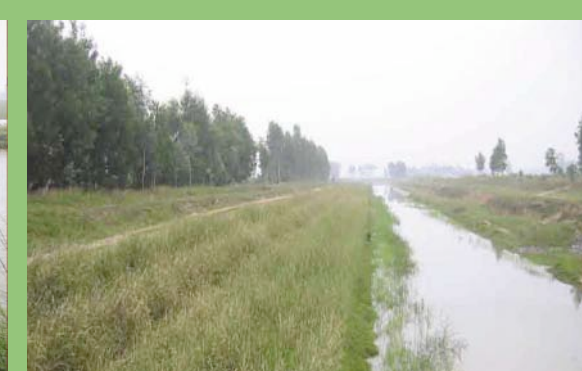
Vietnam - the left hand bank of the canal has been reshaped and stabilized with vetiver, the right bank has yet to be treated.
