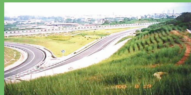
China - expressway stabilization. This cut was prone to massive slip. Stabilization with VS has given complete protection
