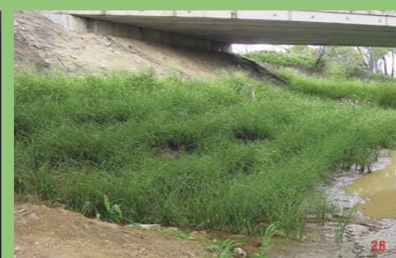
Australia - this river bank and bridge abutment have been stabilized with vetiver. Vetiver is an excellent interface for concrete and soil
