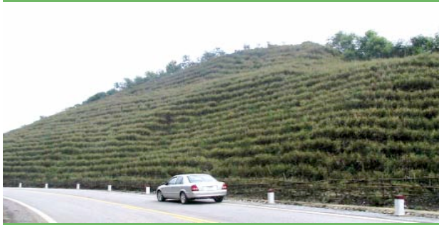
Vietnam: the Ho Chi Minh Highway has been stabilized with vetiver grass. The batters and fills are stable and withstand cyclonic rainfall events
